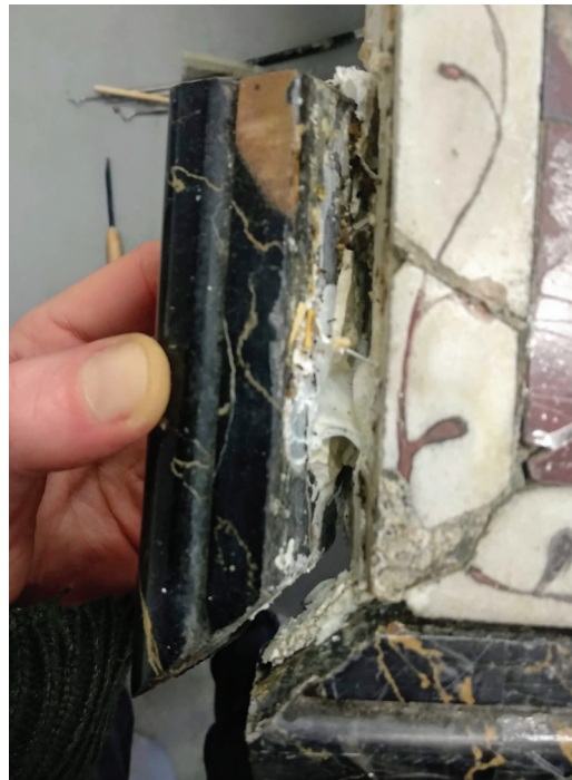
Fig. 11. Removing misaligned mouldings
