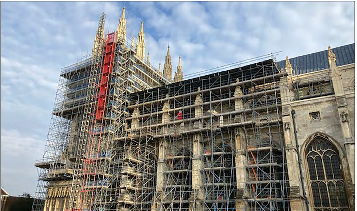
The extent of scaffolding on the South side and West Front of Canterbury Cathedral, needed for the £24.7million 'The Canterbury Journey' National Heritage Lottery Funded project, which sees repair and conservation of the roofs of the Nave and Western Towers; the construction of a new Visitor Centre and shop; new exhibition spaces within the cathedral; new landscaping in the Precincts and the repair, conservation and re-presentation of Christ Church Gate
