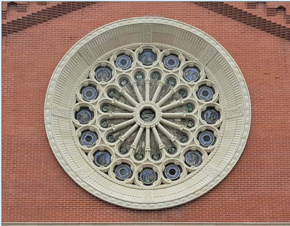
Completed Rose Window cleaning, stabilization, conservation, repair and restoration, including new matching terracotta tracery from Darwen Terracotta Ltd., of Blackburn, UK
