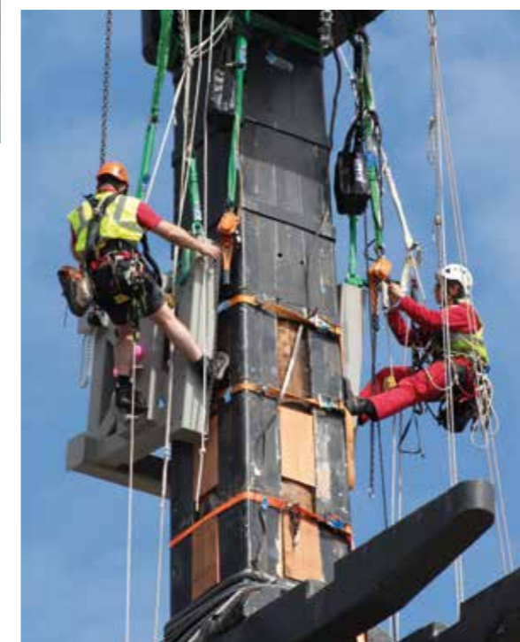
Above: HMS Victory main lower mast removal - installation of upper lift support with riggers
